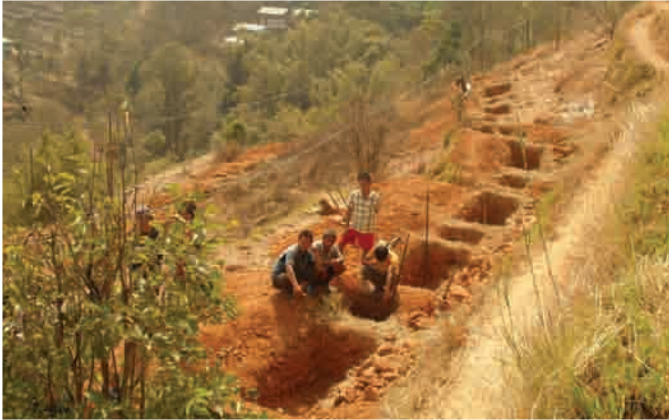
Figure 4: Artificial recharge structures comprising of rows of rectangular staggered contour trenches (2m x 0.8m x 0.6m) with square pits in between for mandarine orange horticulture plantations under construction in privately owned sloping lands in the recharge zone of Malagiri Dhara, Lungchok Kamarey Gram Panchayat, South Sikkim during May 2010
